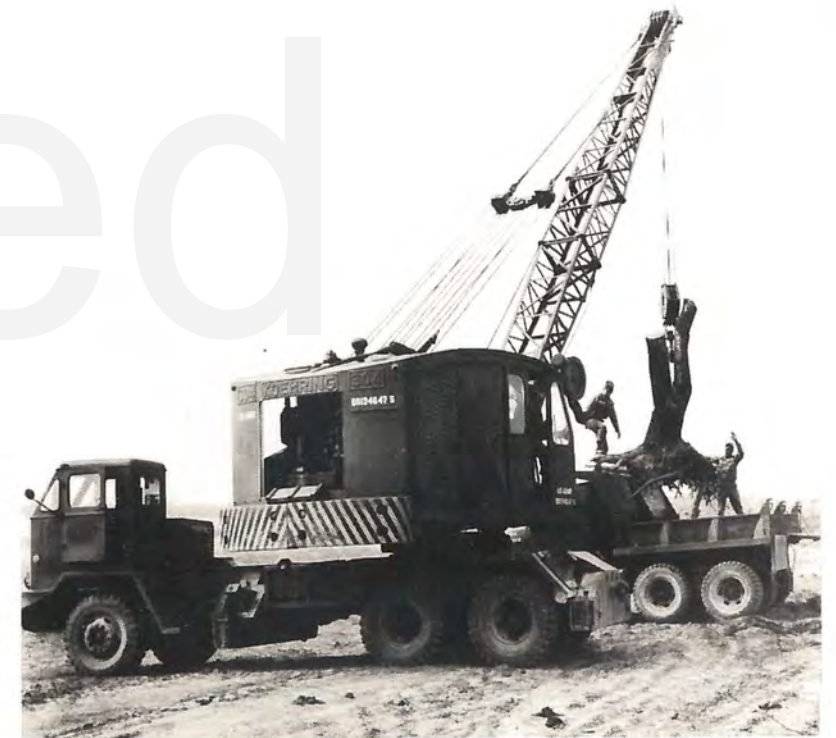
Members of the 22nd Abn. Engr. Co., 187th ARCT load tree stumps, logs and other debris from the 187th DZ while they had the task of clearing the DZ for safer jumps in the future.
