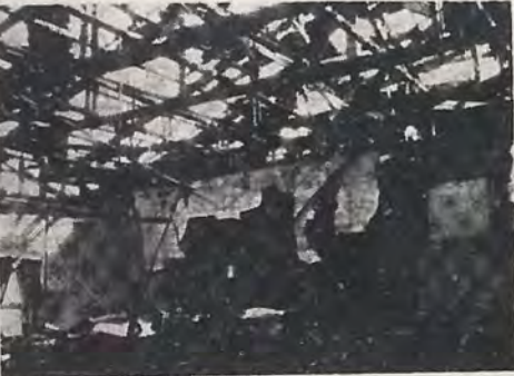
CLOSED FOR REPAIRS: Despite prompt action by the "M" Co. fire alert team, Camp Chickamauga and Beppu fire departments, the Cp. Chick NCO club suffered severe damage last Wednesday morning when it caught fire. (Photo by Humke)
